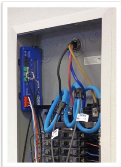
PowerScout 3037 w/RõCoil CTs attached to load
