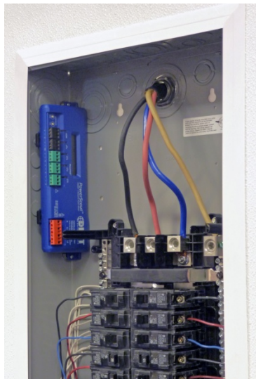
PowerScout 3037 mounted within electrical panel
